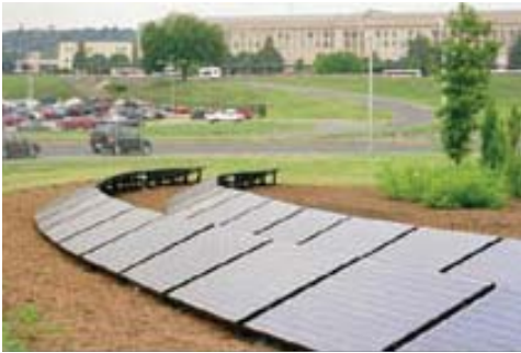
A PV system in Arlington, Virginia, feeds clean energy into the utility grid that supplies electricity to the Pentagon. As a distributed resource, PV puts the power supply at the point of use.
